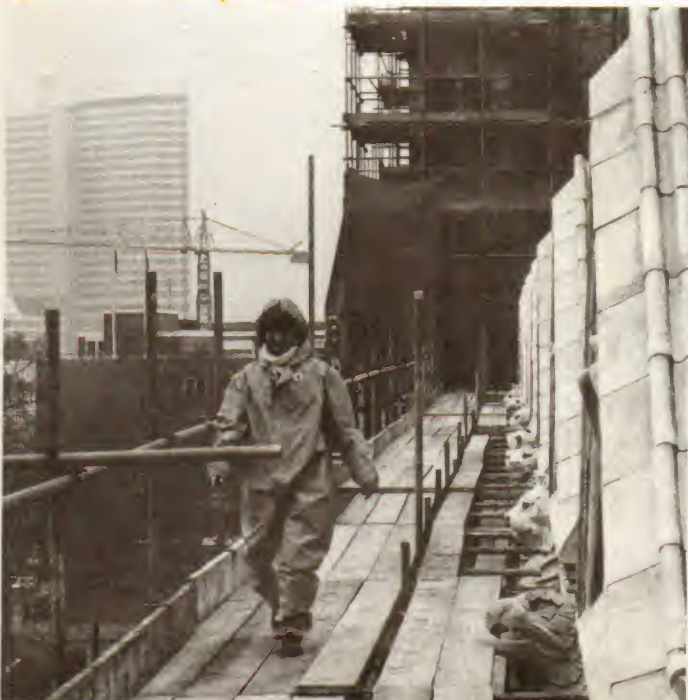
Another view the public doesn't usually see – a whole line up of gargoyles looking like guardsmen on parade.
